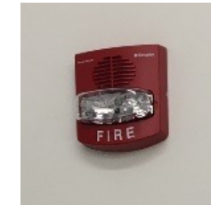
Fire Alarm Indicator
