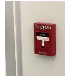
Fire Alarm Pull Station
